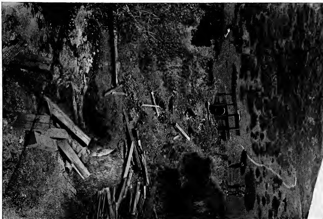
A. Trestle carrying a 30-inch water pipe across Frawley Gulch demolished by shock. R. L. H.
